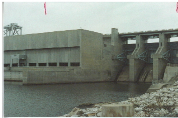
Dam (concrete rebar corrosion)
