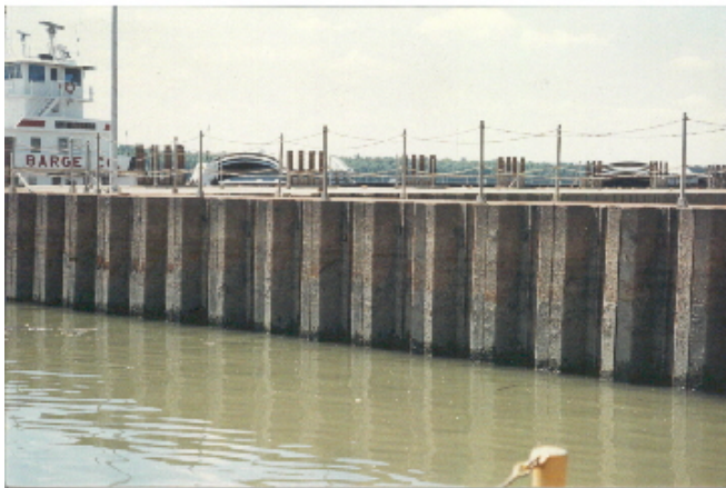
Piling (steel corrosion)
