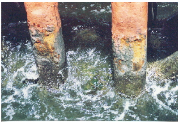
Corroded columns at water line
