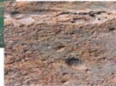
Internal corrosion of oil pipe
