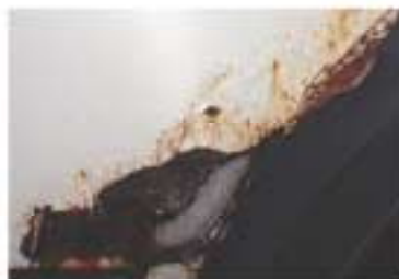
Corrosion under damaged coating
