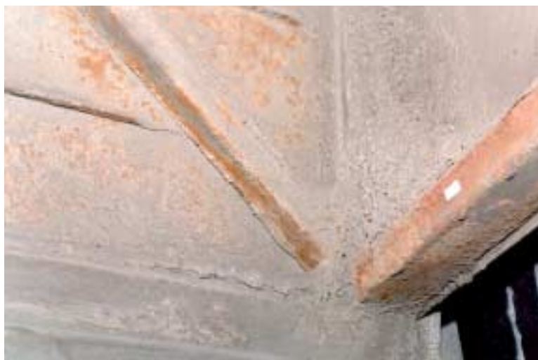
Figure 2. Photograph of poultrice build-up of road contaminants in the wheel area of a bus.
