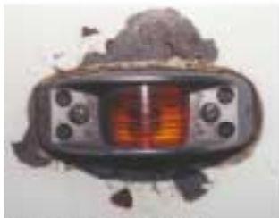
Corrosion at reflector
