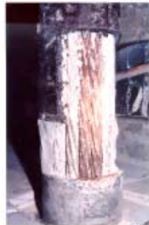
Corrosion in the free length of tendon
