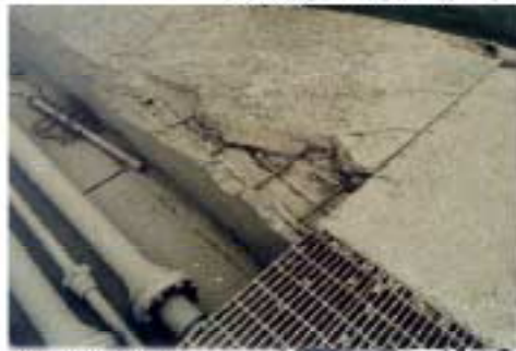
Damaged concrete, exposing rebar
