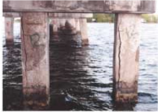
Cracking and spalling of piers in marine environment
