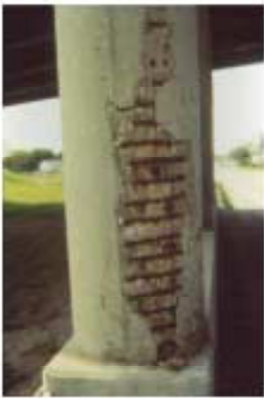
Corroded concrete column
