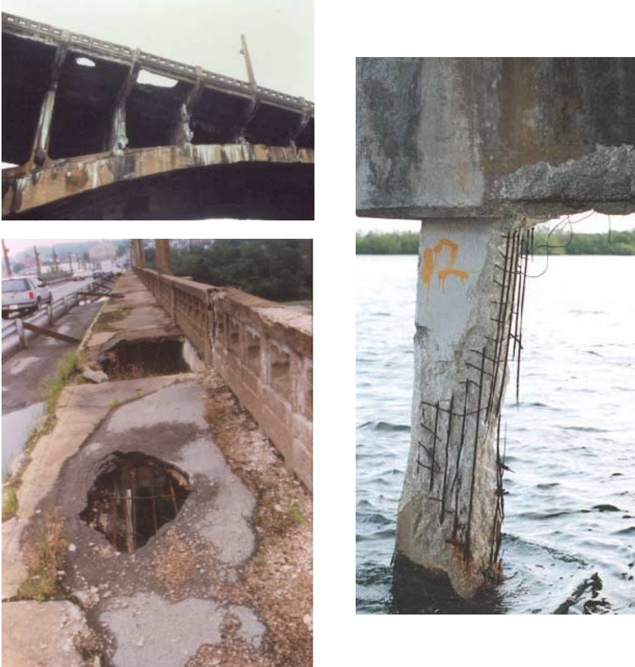
Figure 8. Examples of severe corrosion resulting in deficient bridges.
