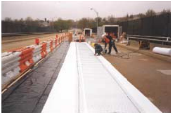
Deck installation of titanium mesh and synthetic felt anode system on bridge deck.
