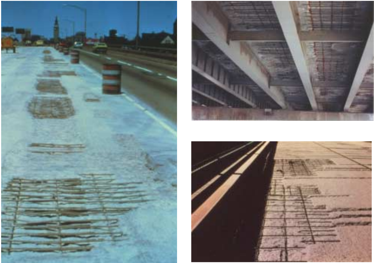
Figure 9. Examples of bridge deck corrosion.
