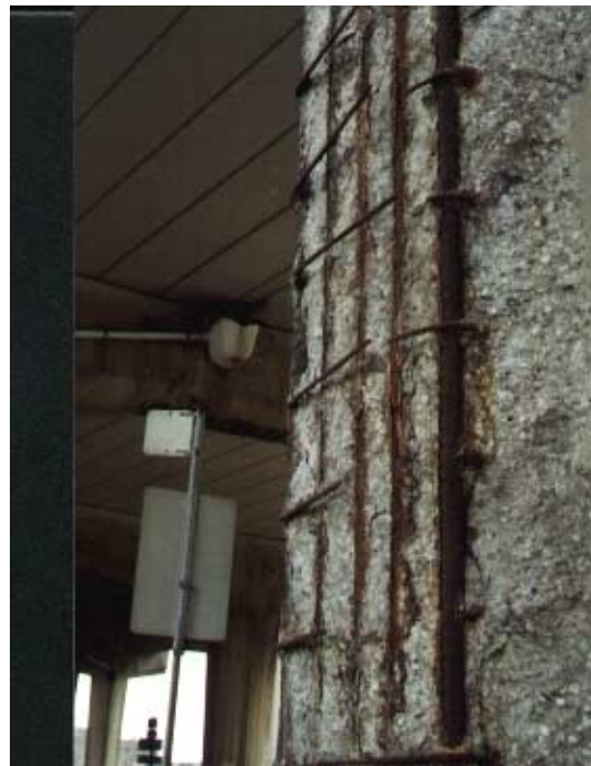
Figure 2. Example of deteriorating bridge element.
