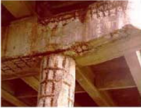
Corroded bridge column
