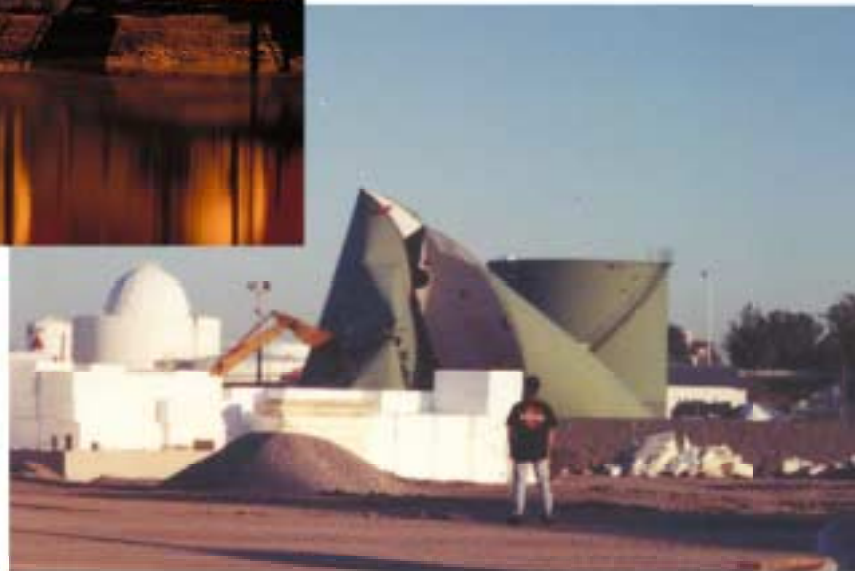
Collapsed storage tank
