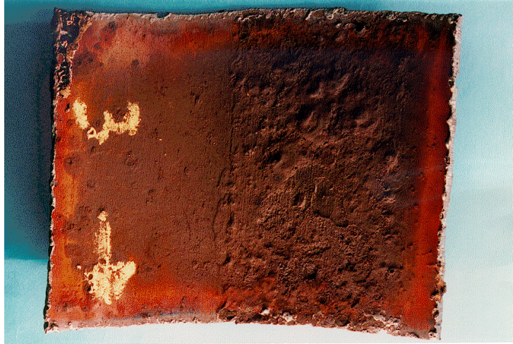
Figure 3. Internal corrosion of a crude oil pipeline.
