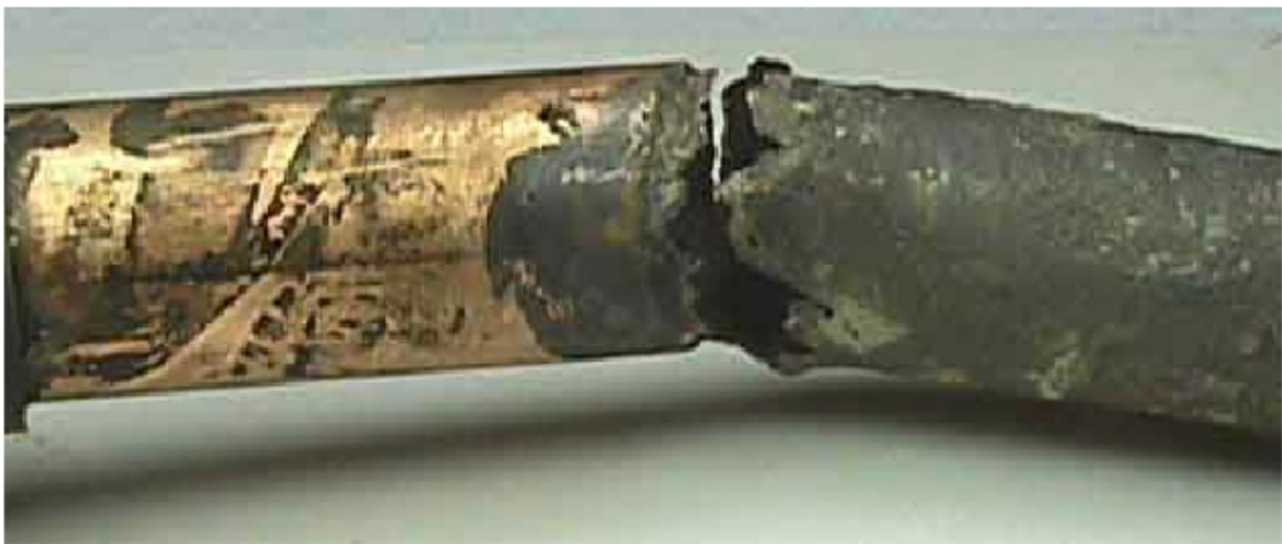
Ruptured gas pipeline
