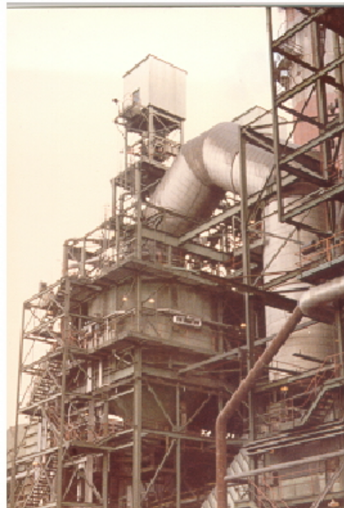
Ducts in power plant
